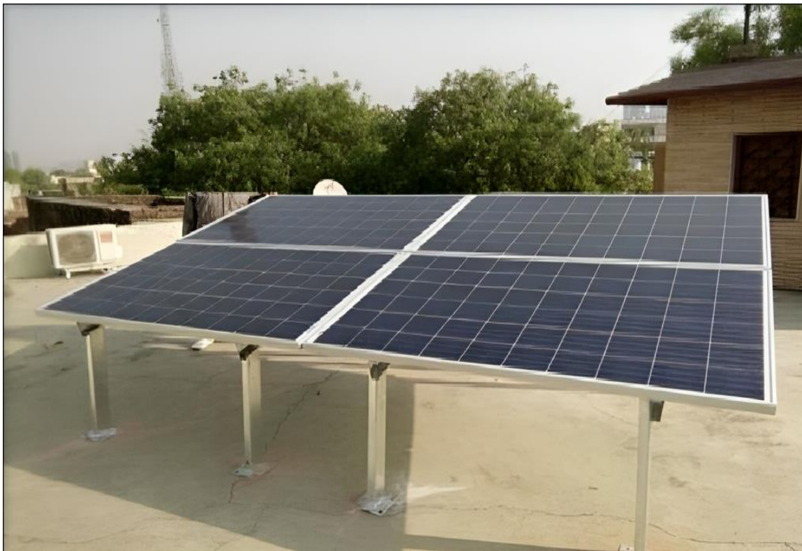
Fig. 1. Photographic view of solar roof top power plant
